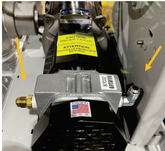
Figure 7-8: Two tubes removed from vacuum pump
