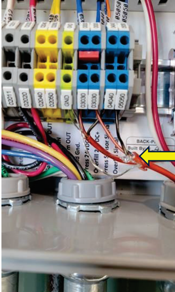
Figure 3-5: GREEN MACHINE Control Panel Connections
