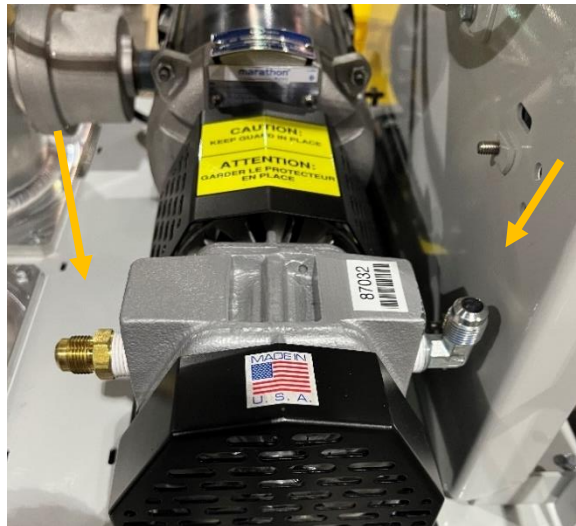
Figure 9-6: Two tubes removed from vacuum pump
