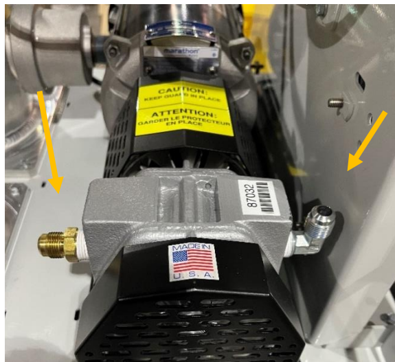
Figure 7-8: Two tubes removed from vacuum pump
