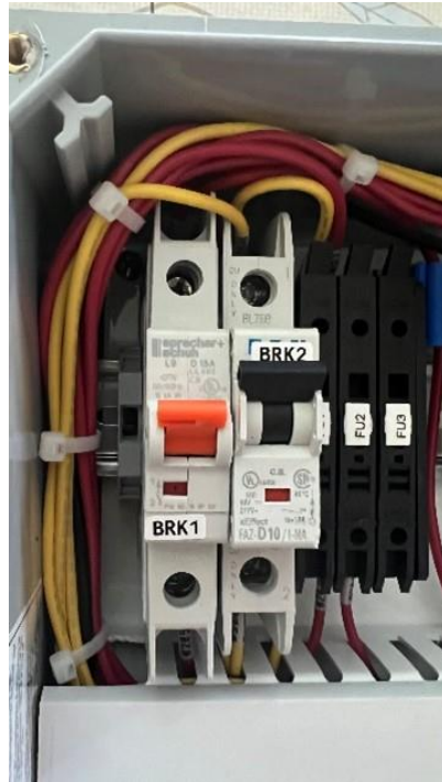
Figure 8-19: Dispenser Bypass Shutdown Breaker (BRK2) is Up (CLOSED)
