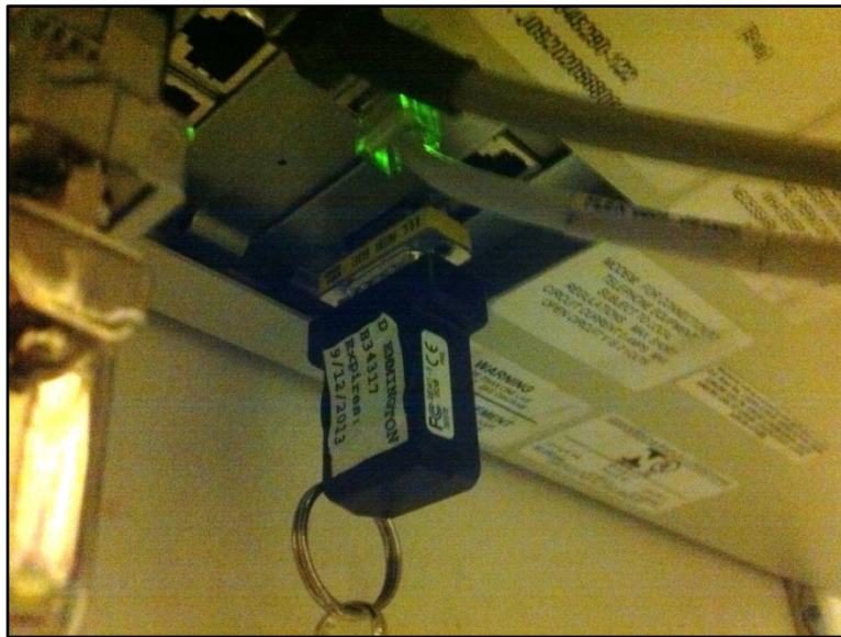
FIGURE 4 Maintenance Tracker Key Plugged Into TLS Console
