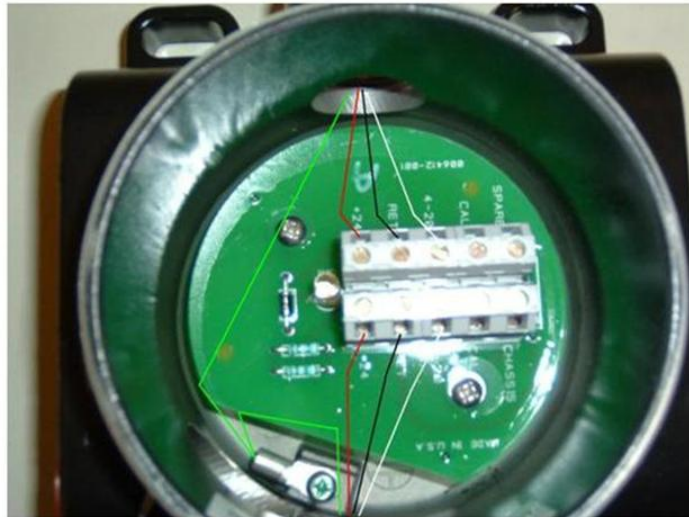
Figure 9: TSP-004 HC Sensor Electrical Junction Box
