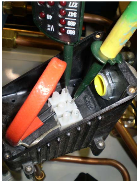
Figure 11: Heat Trace Circuit Test
